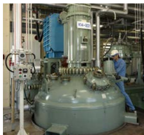
Reactor: 8000 L Glass-lined
